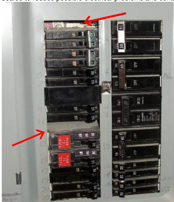
Physical damage --- Physical damage was noted and should be repaired. Location: Cut insulation on wire
